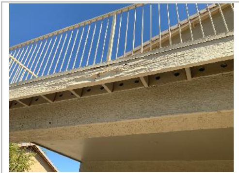
Water damage back porch fascia
