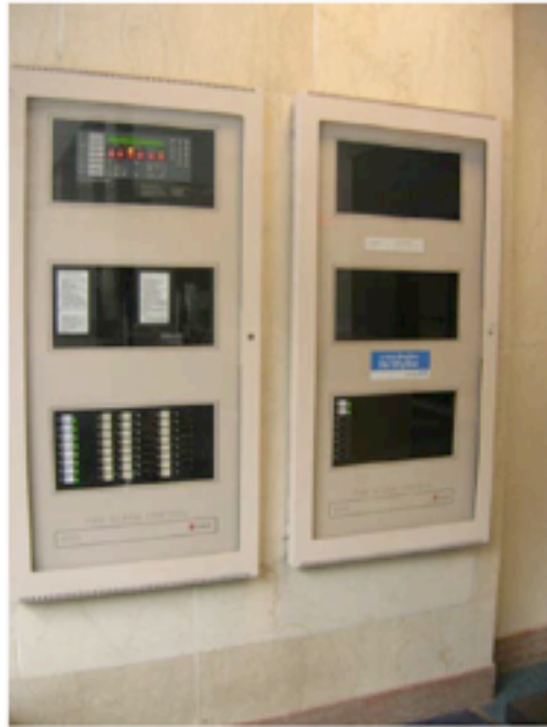
Fire & Security System
